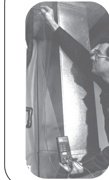
FIGURE 42 TEMPERATURE RISE MEASUREMENT
